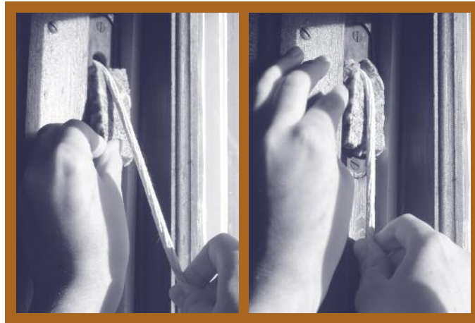
A piece of foam carpet pad can be used to block drafts around the pulleys of older double-hung windows. Pull the rope or chain out a bit, insert the foam pad, and release the rope or chain so the weight holds the pad in place, blocking the opening around the pulley.
